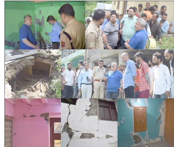
Deputy Commissioner Doda, Vishesh Mahajan and SSP, Abdul Qayoom today toured Sub Division Gandoh to ascertain the situation after the 5.4 magnitude earthquake that shook the district the previous day.
